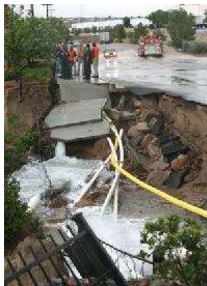
People looked down at a giant sinkhole created from flood waters at Esther Lama and Henry Brennan in East El Paso Friday. (Rudy Gutierrez / El Paso Times)
